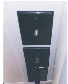
CEILING MOUNTED ANTENNA POWER SUPPLY
