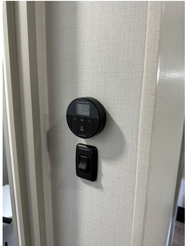
The bedroom thermostat is located just inside the bedroom door on the bathroom wall.
